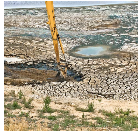
Figure 2 Sediment management infrastructure in Baltimore, Maryland. Here, machine operators at the Cox Creek Dredge Material Containment Facility are undertaking crust management through using a long-arm excavator, evapotranspiration, and hydrostatic pressure.
