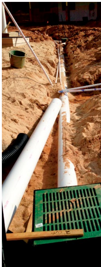
Example of a surface drainage system, which may be the only viable, long term solution.
