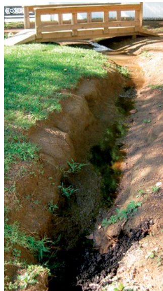
Poor drainage at childcare centers can lead to erosion and unseemly gullies.
