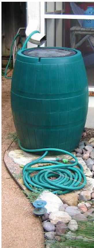
Rain barrel connected to a hose intercepts run-off and conserves for later irrigation.
