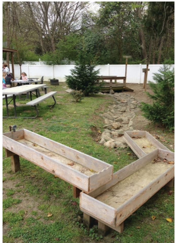
Stream bed remediation of erosion gully. Stones are cemented into channel. Water drains from a series of "hands-in" water troughs fed by faucet.
